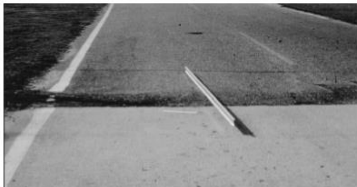
Figure 146: Shoving Source: FHWA, 1998
