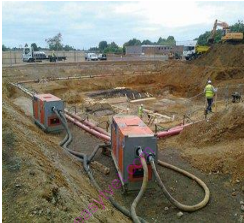
Fig. 33 a picture of well point method of dewatering Ref. a adopted from: sldpumpspower.com
