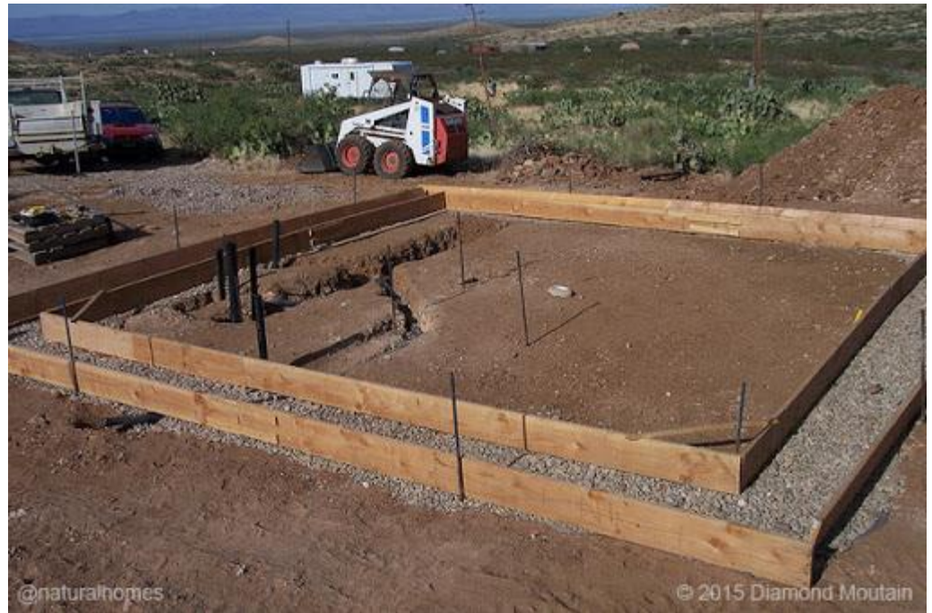
Figure 44 : A picture of foundation formwork read to receive concrete adopted from: shutterstock.com
